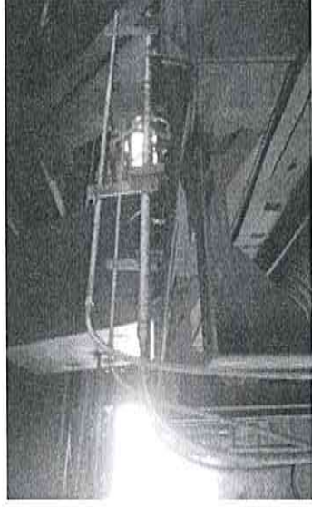
Fixed type DS system for coal Conveyor
