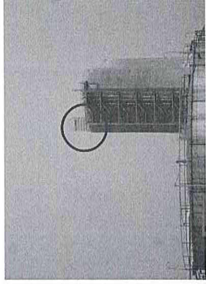
Bag Filter installed at Ash silo
